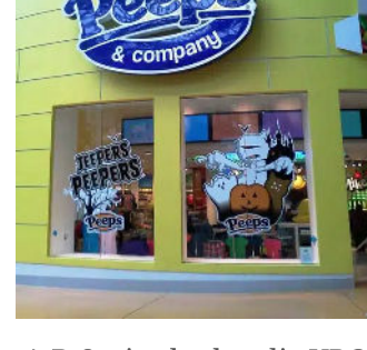
A D Series hydraulic VRC lift serves the Peeps & Co. store at the Mall of America.
